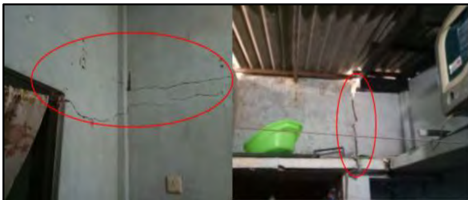
Figure 2: Wall Cracks in Damaged Houses
